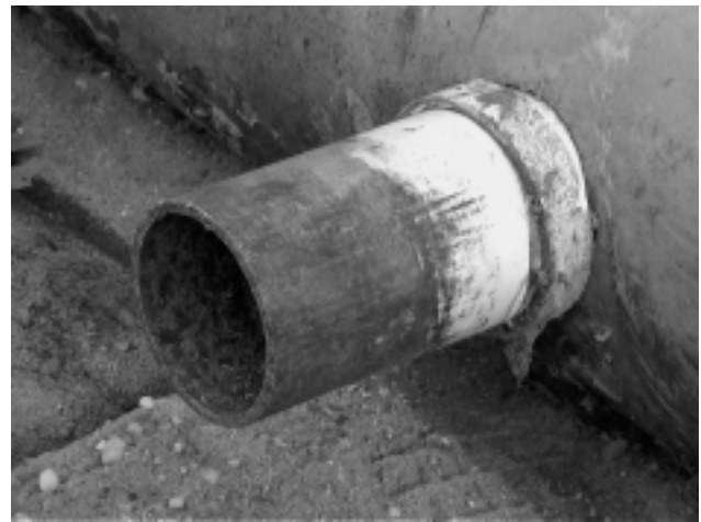
Figure 4 – Four inch nipple in trunkline
